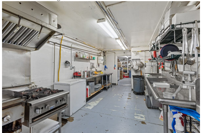
Commercial Kitchen — Range & Hood
