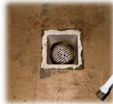
Floor drain for sink
