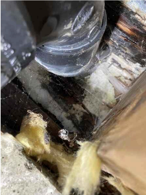
***This is an Example picture*** This is an example of what it could look like under the floor if it is not addressed
