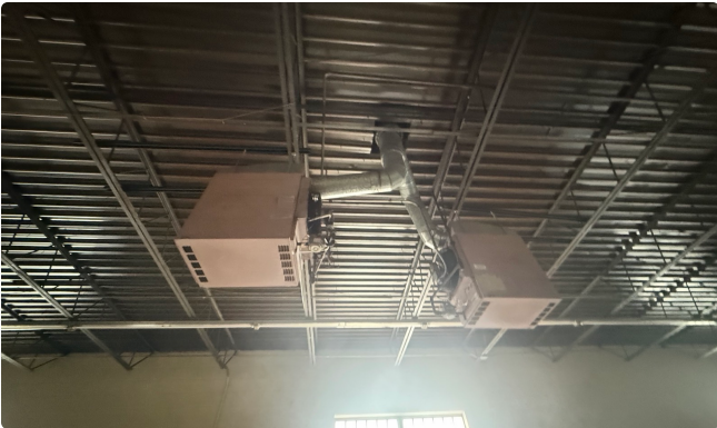
Overhead warehouse heaters
