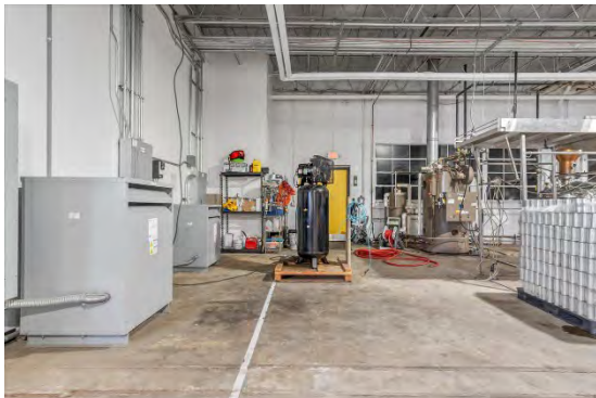
View of Inside Power
