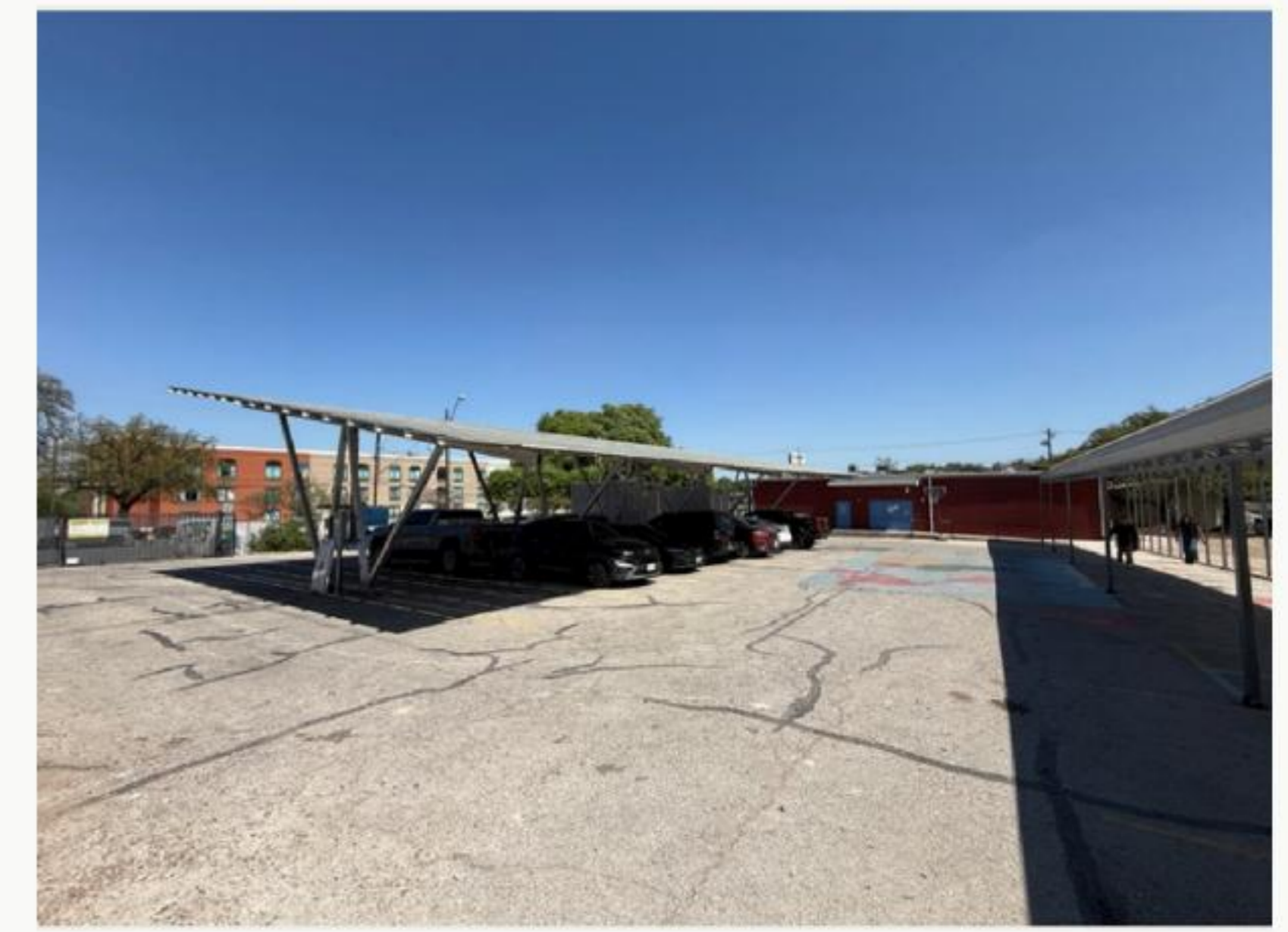
Solar carport — rear lot
