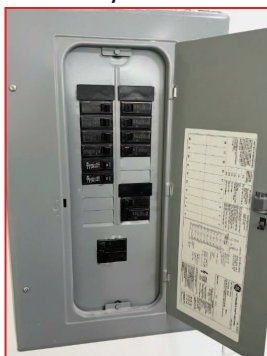
Electrical Panel, Cover On
