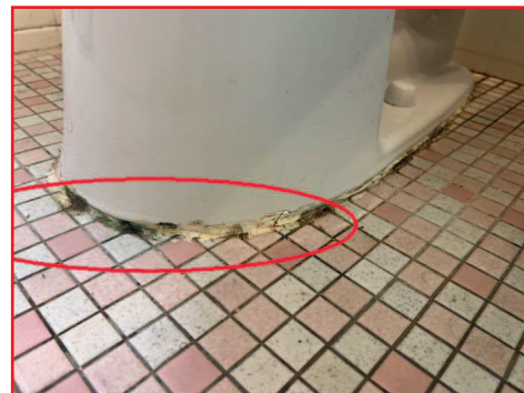
Possible mold noted
