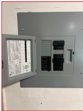
Electrical Panel, Cover On
