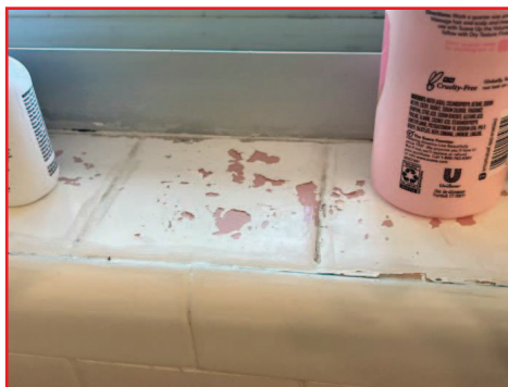
Painted Tile Peeling
