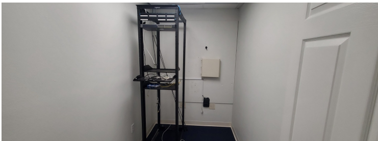
SERVER / IT ROOM
