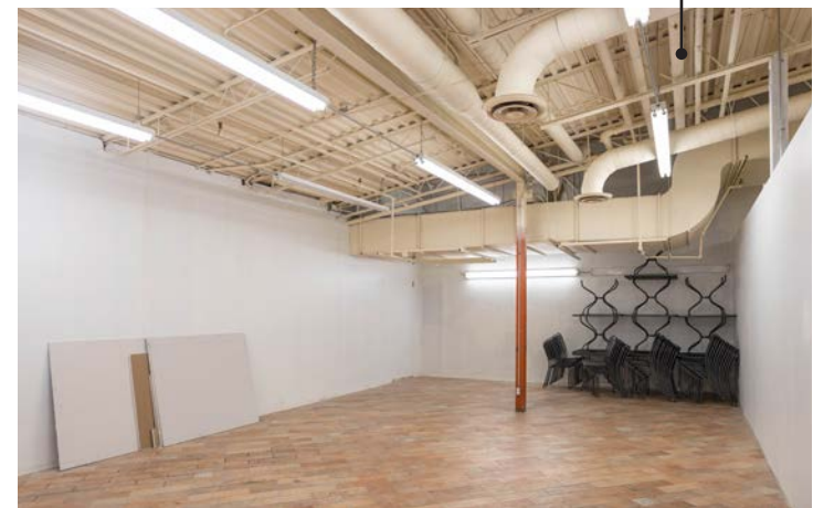
Easily accessible ventilation system
