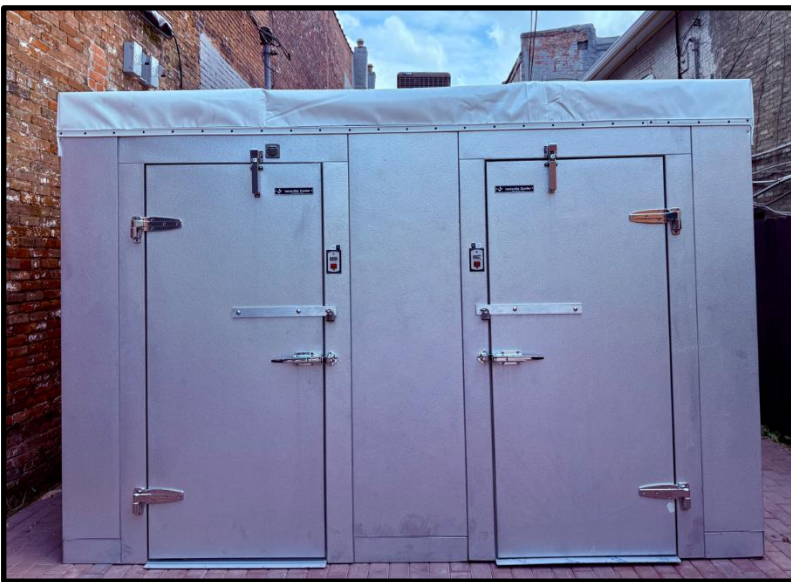
PICTURE 2: 12X12 WALK IN REFRIGERATION & FREEZER
