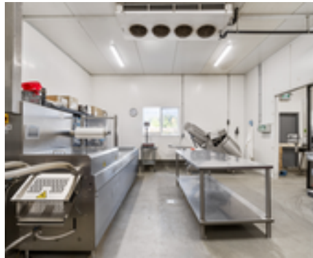
Processing area — cold-chain equipment
