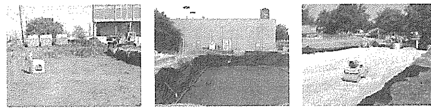
Excavate bed and prepare subgrade per engineer's plans. Place non-woven geotextile over prepared bed and up excavation walls. Install underdrains if required. Place clean, crushed angular stone foundation @ (150 mm) min. Contractor achieve a flat surface.
