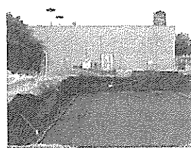
Place non-woven geotextile over prepared soil and up excavation walls. Install underdrains if required.
