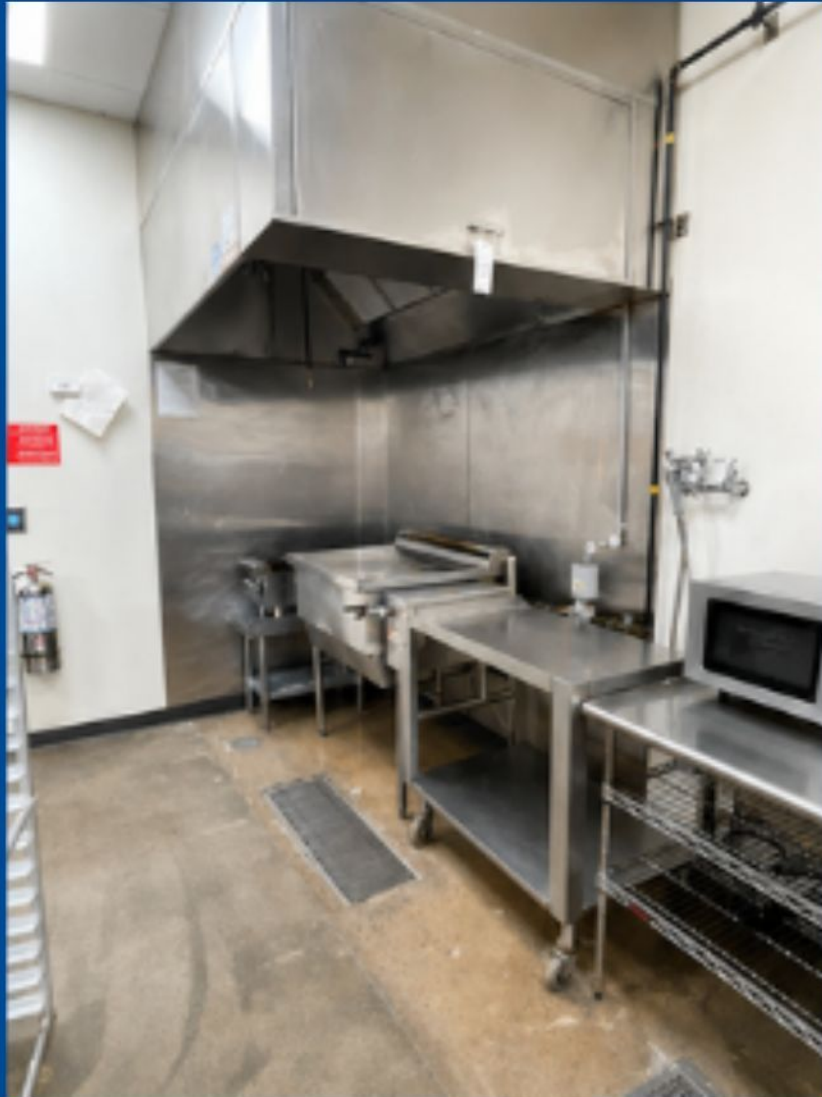
Commercial Ventilation Hood
