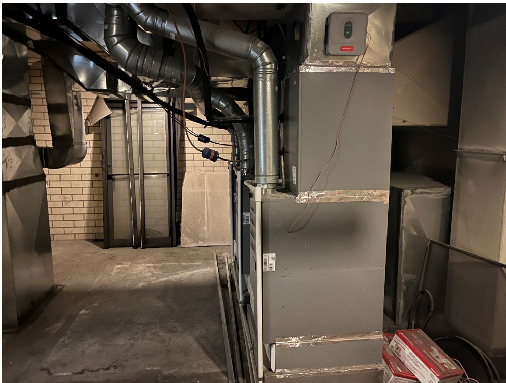
Photo 6 - View of the furnace, which is located in the basement.
