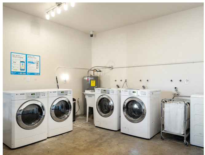
ON-SITE COIN-OP LAUNDRY — ANCILLARY INCOME
