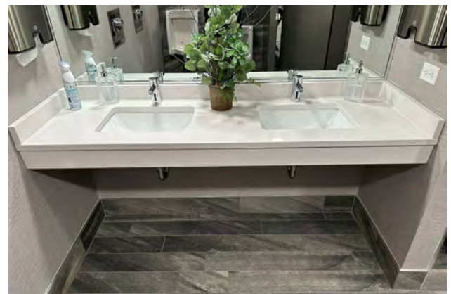
Common area bathrooms
