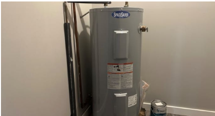
COMMON TANK — SERVES THE LAUNDRY ROOM ONLY
