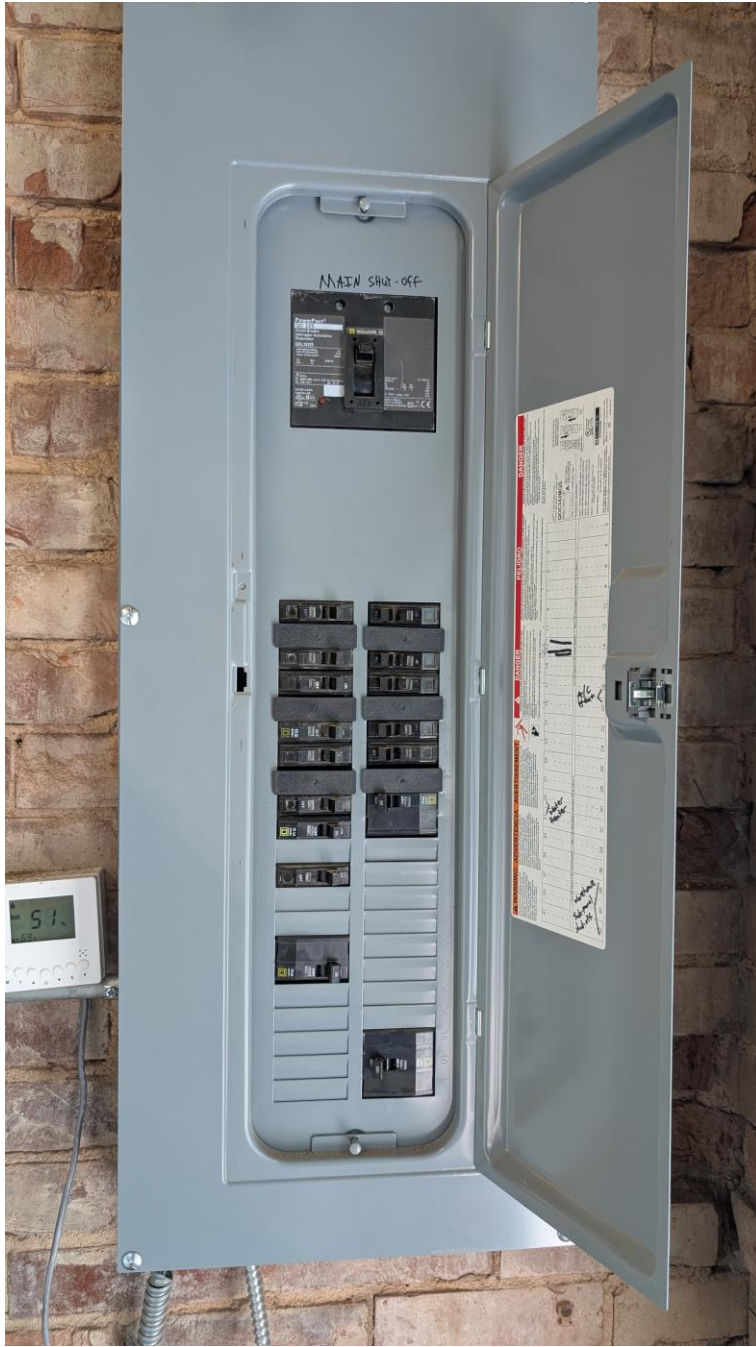
Main electric panel
