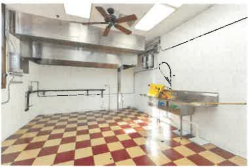
Kitchen with vent hood
