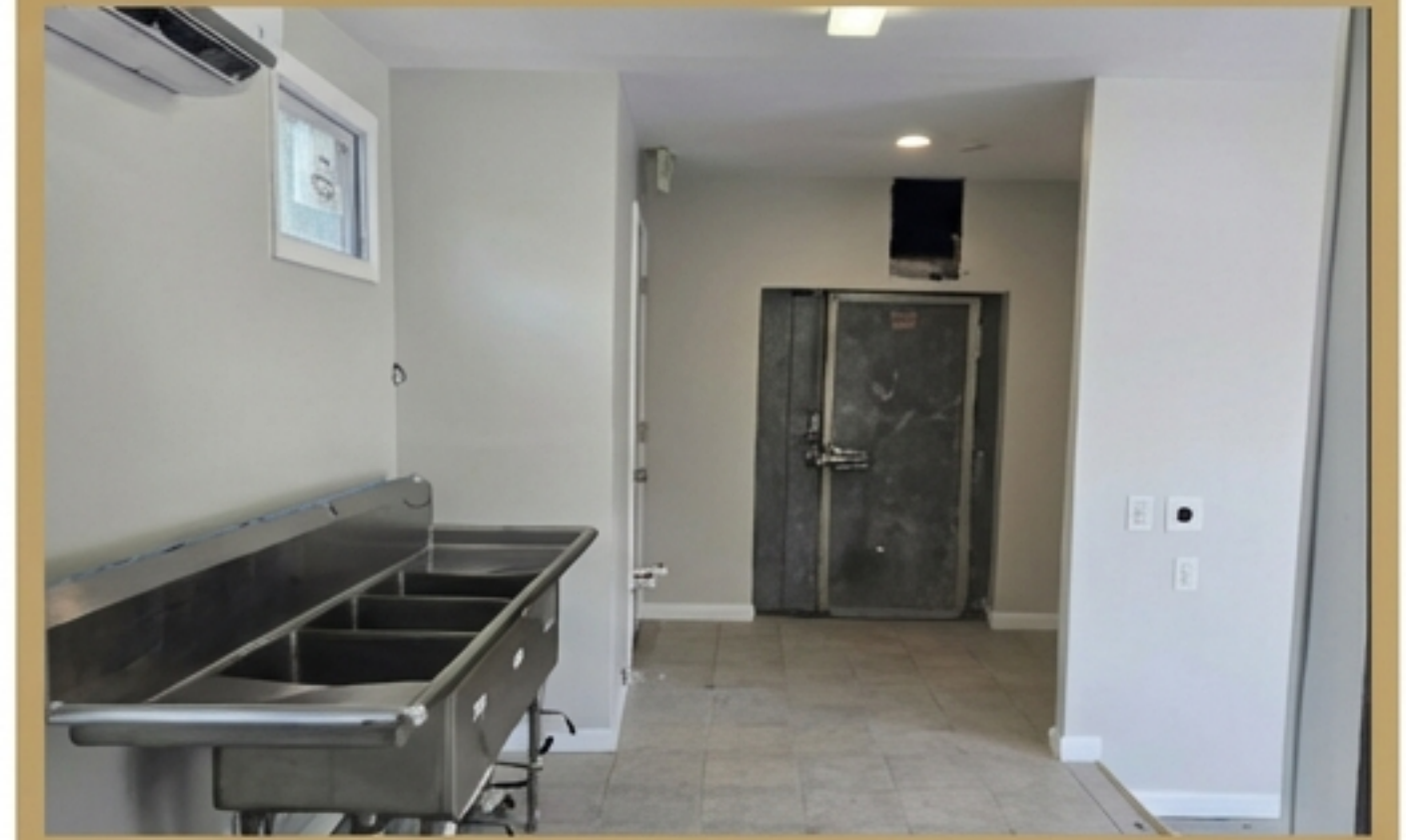
New mechanicals and utility installations.
