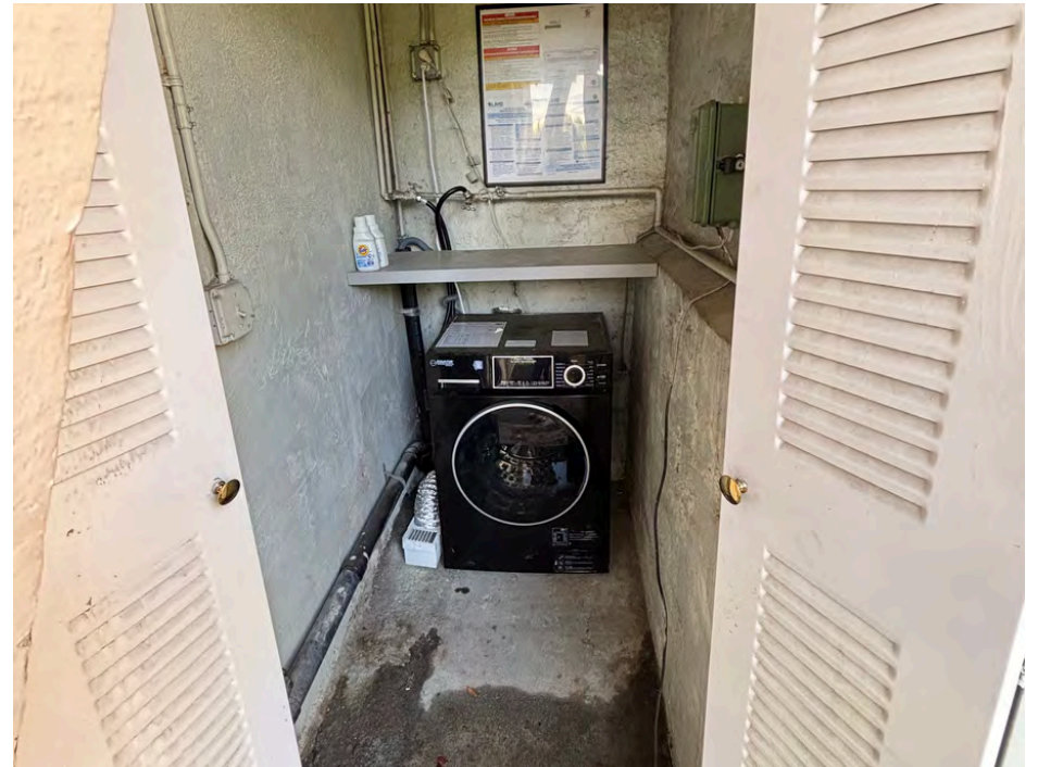
Washer & Dryer Outside of 3055
