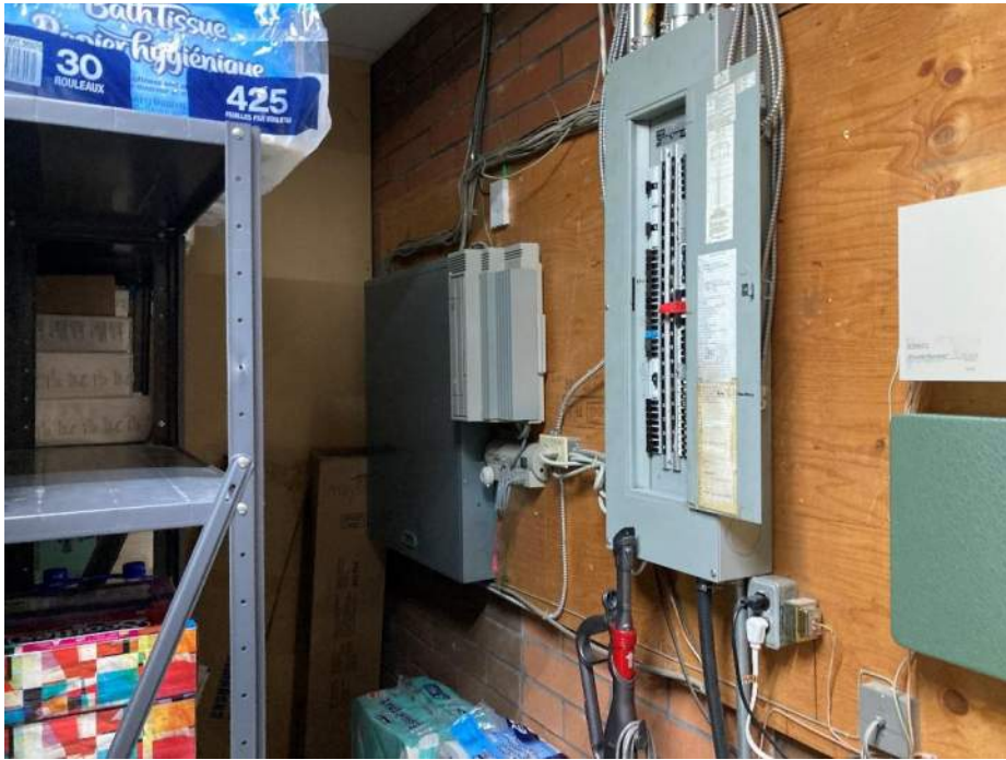
Photograph No. 11. View of electrical panel located within utility closet for Kern's Furniture.
