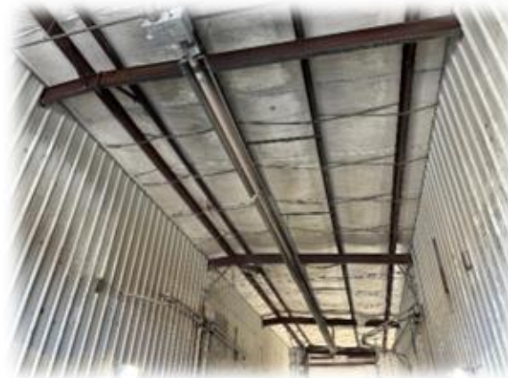
Radiant Heating In Car Wash Bays
