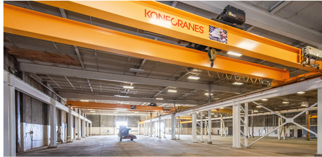
Unit A: Two (2) 10-Ton Top-Running Girder Bridge Cranes (Separate from Previously Pictured Cranes)
