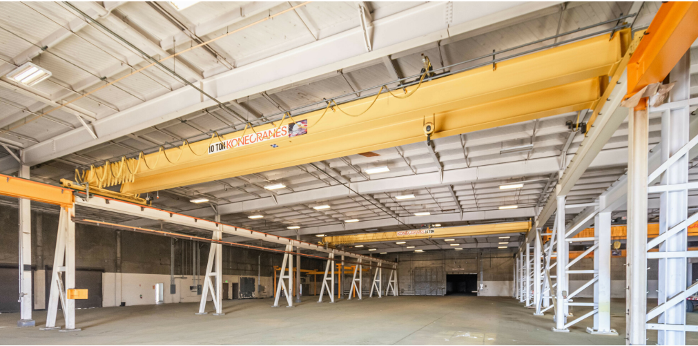
Unit A: Two (2) 10-Ton Top-Running Girder Bridge Cranes
