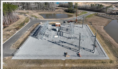
On-Site Palmetto Electric Substation
