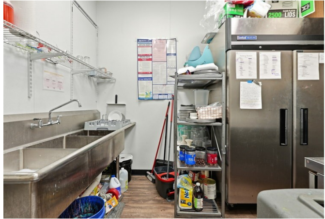
Rear wash and prep room with utility plumbing and floor drainage
