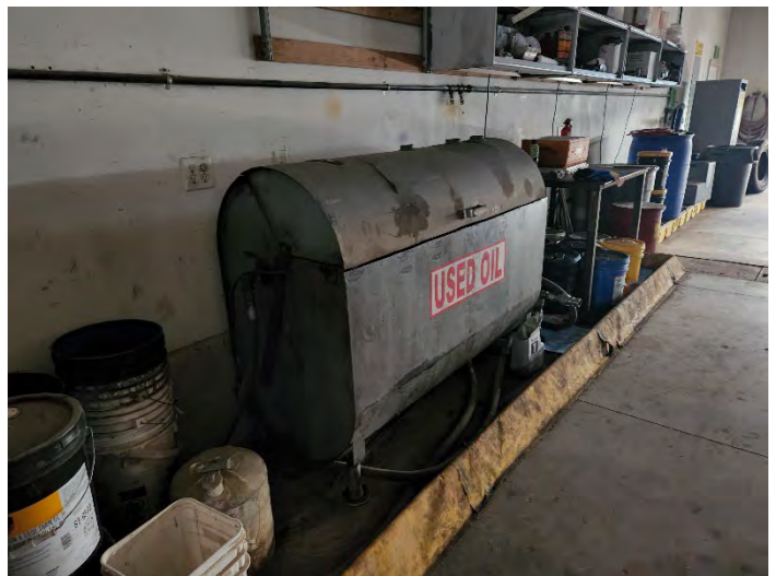
16. 250 gallon used oil tank
