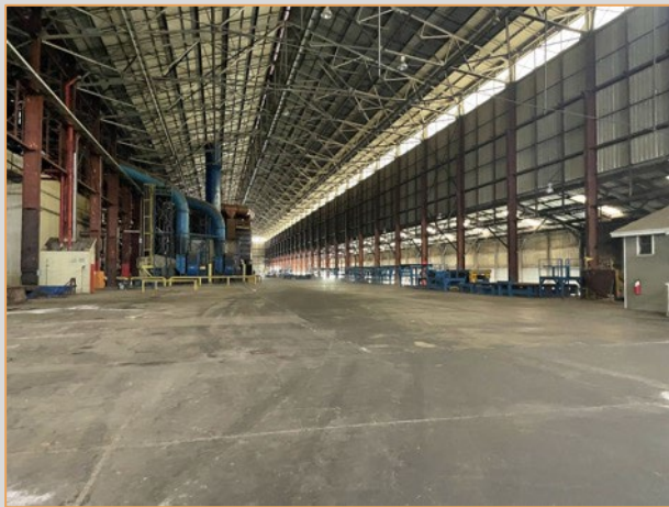
Main plant interior
