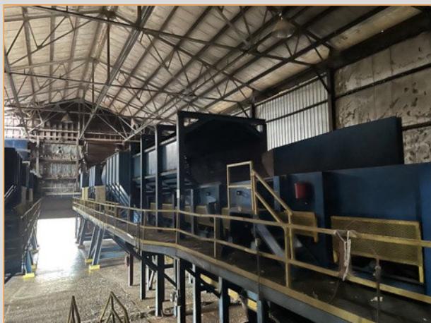
Main Plant Interior
