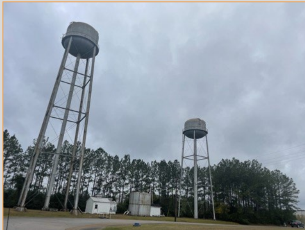
On site water supply
