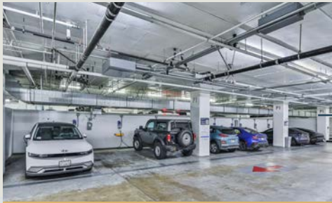
Parking with EV Charging Stations
