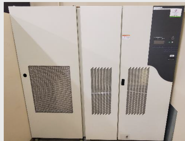
UPS Backup System
