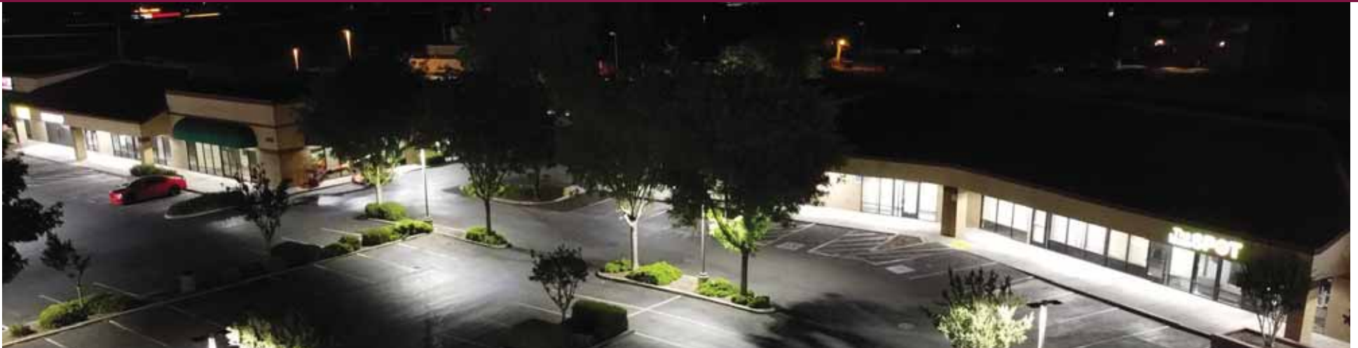
NEW LED OUTDOOR LIGHTING UPGRADED
