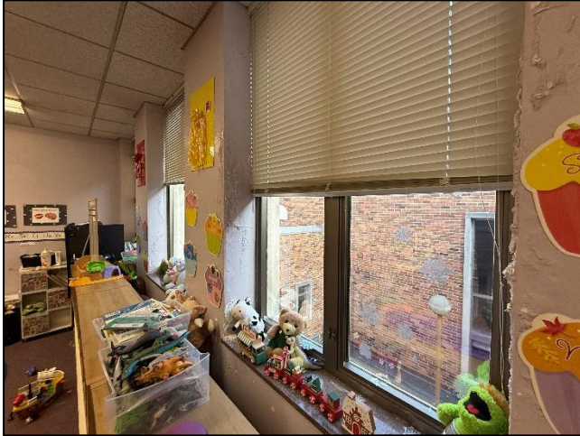
Interior damage on window
