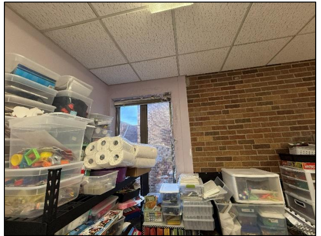
Interior damage on window
