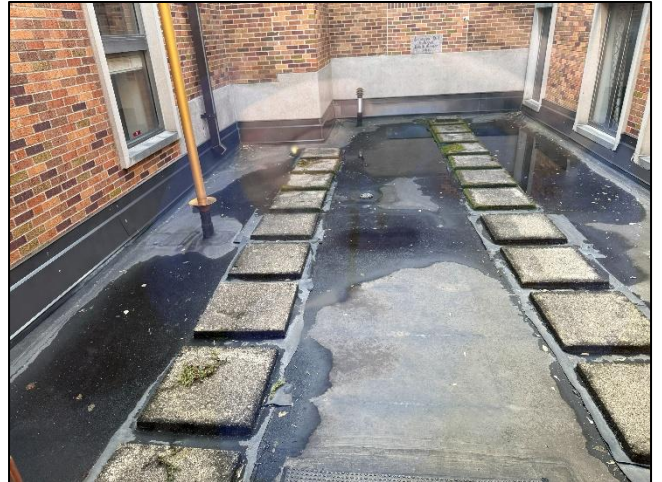
Roof damage area
