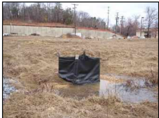
Catch basin within site interior is part of site drainage system, and is protected by silt fence as part of site construction activities.
