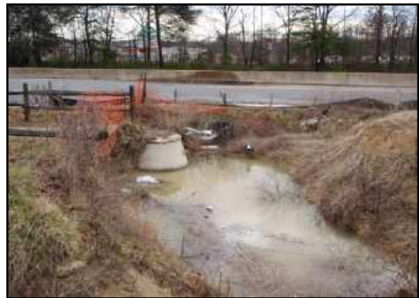
End of drainage gully at northeast corner of the site.
