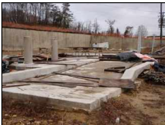
Concrete pad on subject property, presumably placed as the foundation for a concrete plant.
