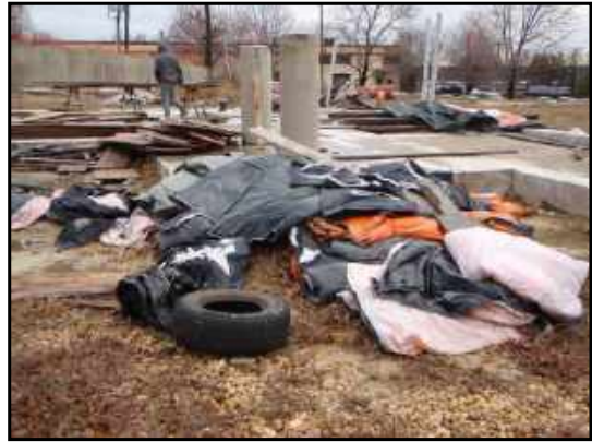
Construction materials and debris at concrete pad.
