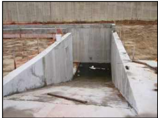
There is a concrete-lined and constructed pit on the west side of the concrete pad, which presumably was to provide access beneath aggregate feed bins for the concrete plant. This pit was observed to be holding approximately 1.5 feet of water.
