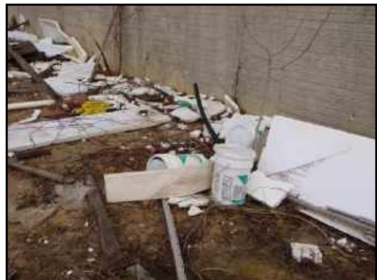
Debris at northwest site corner includes buckets and insulating material.
