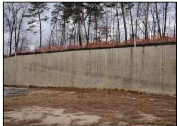
Retaining wall on western side of site. Interstate highway Route 95 is located directly west of the site, beyond the trees above the retaining wall.
