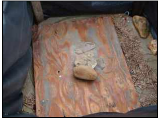
Cover over manhole that is part of on-site drainage system.
