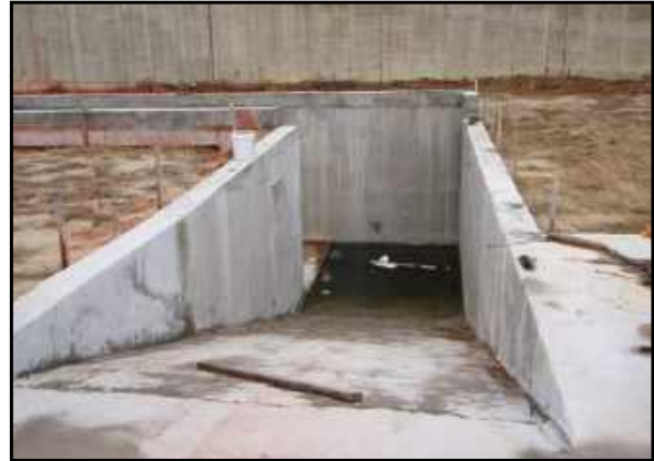
There is a concrete-lined and constructed pit on the west side of the concrete pad, which presumably was to provide access beneath aggregate feed bins for the concrete plant. This pit was observed to be holding approximately 1.5 feet of water.
