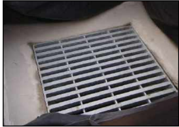
Catch basin associated with on-site drainage system.
