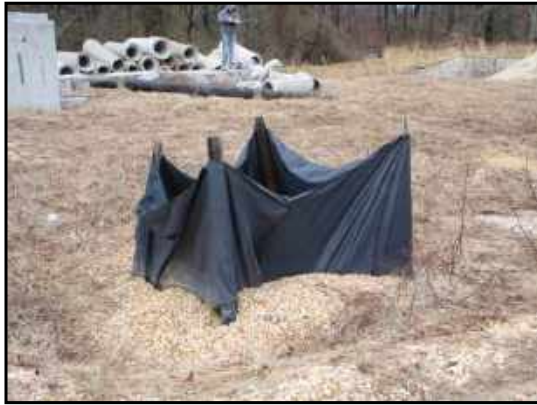
Catch basin on site, protected by silt fence.
