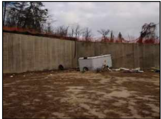
Retaining wall on western side of property, and small storage trailer at northwest corner of site.
