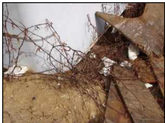
Bottom of small storage trailer at lower end. No staining of ground around the perimeter of the storage trailer was observed.
