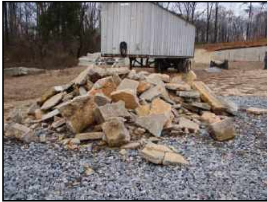
There is a pile of broken concrete rubble on the entrance drive. Storage trailer in background.
