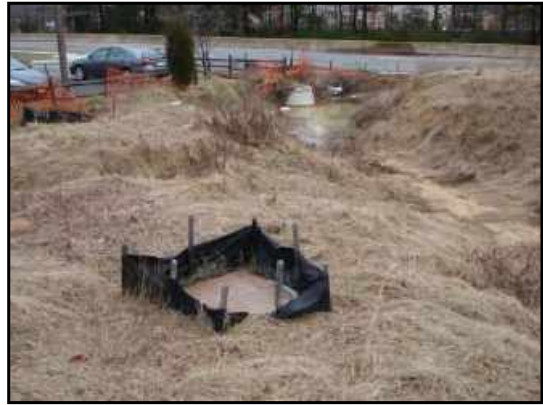
View of gully and drainage at the northeast corner of the site.
