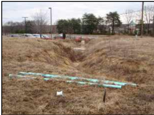
Drainage gully on northeast corner of subject property. The origin of this gully is unclear, but may have been caused by site excavation.
