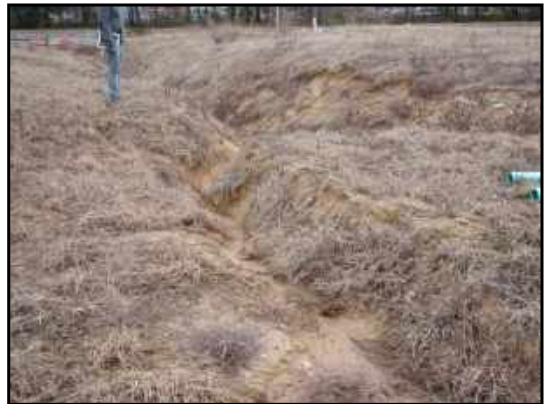
Erosion at top of gully on northeast corner of property.
