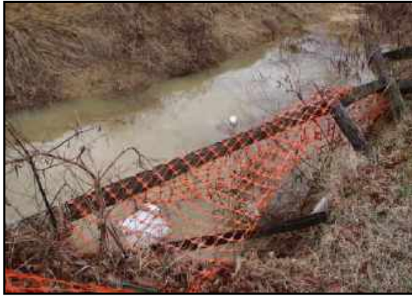
Water ponded within gully at northeast corner of site.
