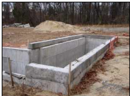
Concrete-lined pit, presumably constructed as part of aggregate feed bin system for concrete plant.
