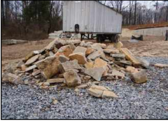
There is a pile of broken concrete rubble on the entrance drive. Storage trailer in background.
