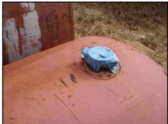
Tape used as a cap on the smaller (100-gallon) aboveground tank.
