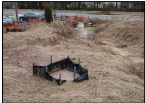
View of gully and drainage at the northeast corner of the site.
