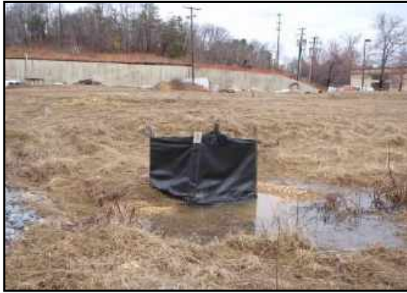
Catch basin within site interior is part of site drainage system, and is protected by silt fence as part of site construction activities.
