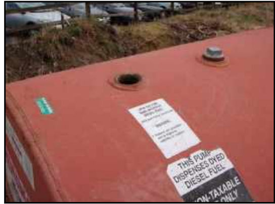
Open cap on 1,000-gallon aboveground storage tank. This tank is marked to contain off-road diesel fuel, and contains a small volume of liquid with a petroleum odor.
