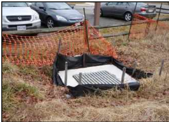
Catch basin protected by site fence at the northeast corner of the site.
