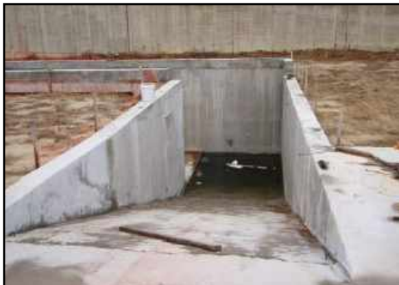
There is a concrete-lined and constructed pit on the west side of the concrete pad, which presumably was to provide access beneath aggregate feed bins for the concrete plant. This pit was observed to be holding approximately 1.5 feet of water.
