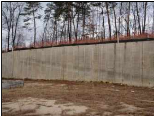
Retaining wall on western side of site. Interstate highway Route 95 is located directly west of the site, beyond the trees above the retaining wall.
