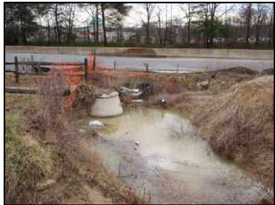
End of drainage gully at northeast corner of the site.
