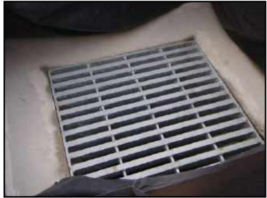
Catch basin associated with on-site drainage system.
