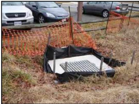
Catch basin protected by site fence at the northeast corner of the site.
