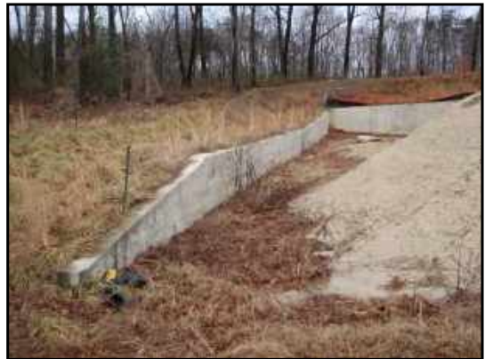
The western side of the site includes a large retaining wall, which extends partially along the southern side of the site (shown here) and the northern site boundary.
