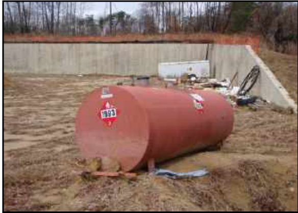
Aboveground storage tank, approximately 1,000-gallons in size (unmarked as to size) on site at central-northern portion of site. The tank appears to contain some petroleum product inside, with the cap off it may also be receiving rainfall. The tank appear
