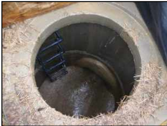
Manhole that is part of on-site drainage system.
