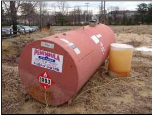
Large 1,000-gallon aboveground tank and adjacent 55-gallon drum on north side of site.
