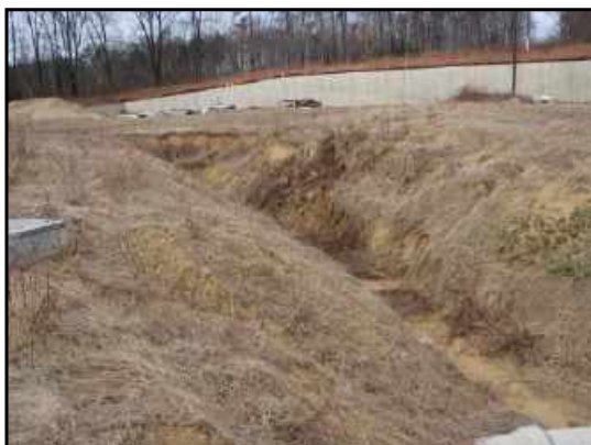
Drainage gully on site, which may have been excavated, looking to west side of site.
