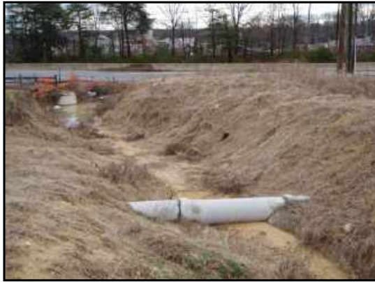
Gully on subject property, looking towards northeast corner of site. Drainage pipe is visible crossing the gully, which appears to be part of the on-site drainage system.
