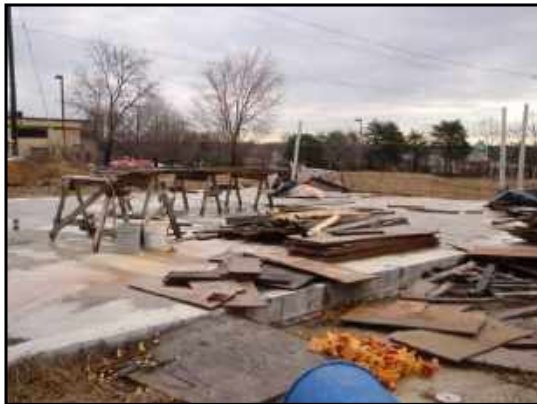
Construction materials (such as wood) on concrete pad.
