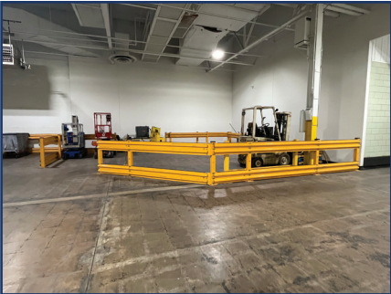
FORKLIFT CHARGING STATION
