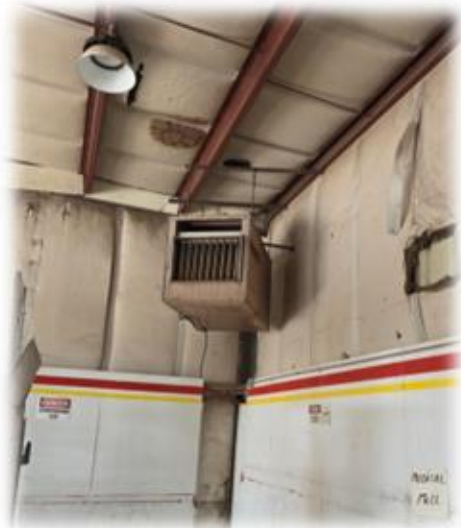
Suspended Heat in Detail Shop
