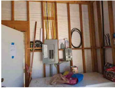
Garage Electric Panel
